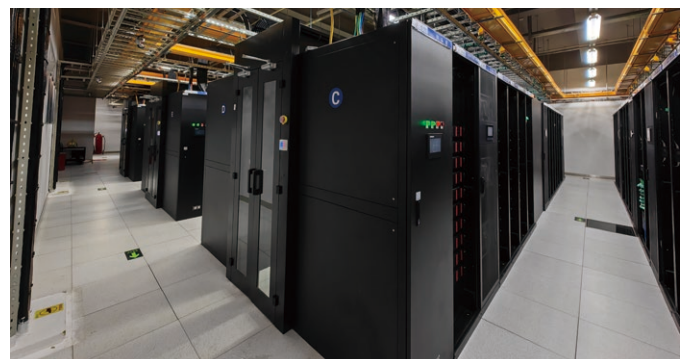
© A green and energy-efficient server room of Hubei Mobile
