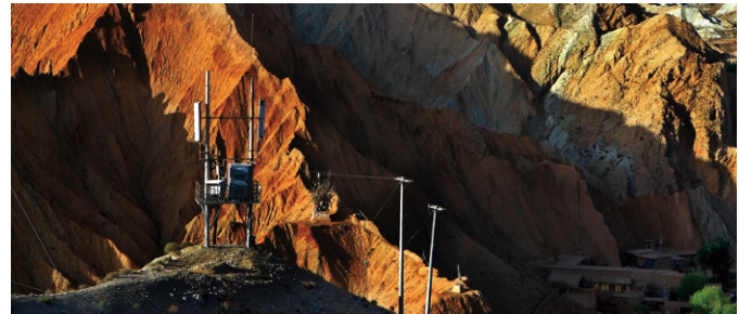
© Gansu Mobile built a base station in Nantai Village, Linze County, Zhangye City, to improve access to communication services in remote mountain villages
