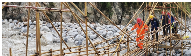
© An 8-person advance team from Sichuan Mobile hiked to the Hailuogou Scenic Area to repair base stations
