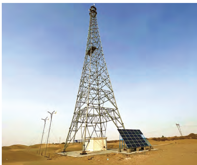
Building solar energy base station in Xinjiang.
