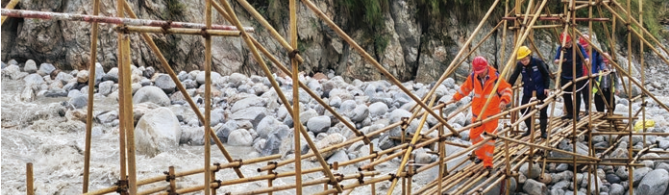
© An 8-person advance team from Sichuan Mobile hiked to the Hailuoguo Scenic Area to repair base stations
